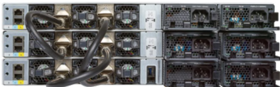
Figure 5. Cisco Catalyst 9300 Series switch stack units
